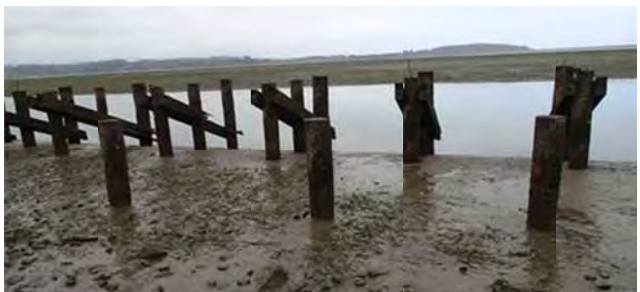
Derelict wharf along Channel in south Humboldt Bay at the south end of Fields Landing. Decking was removed from the final remaining portions of the wharf as late as 2009. The shade removal exposed areas of the intertidal to recruitment of eelgrass. As much as 1.8 acres of bay coverage was removed from 2005 to 2009 with the result being recruitment of approximately 0.5 acres of eelgrass back on to the exposed mudflats.
