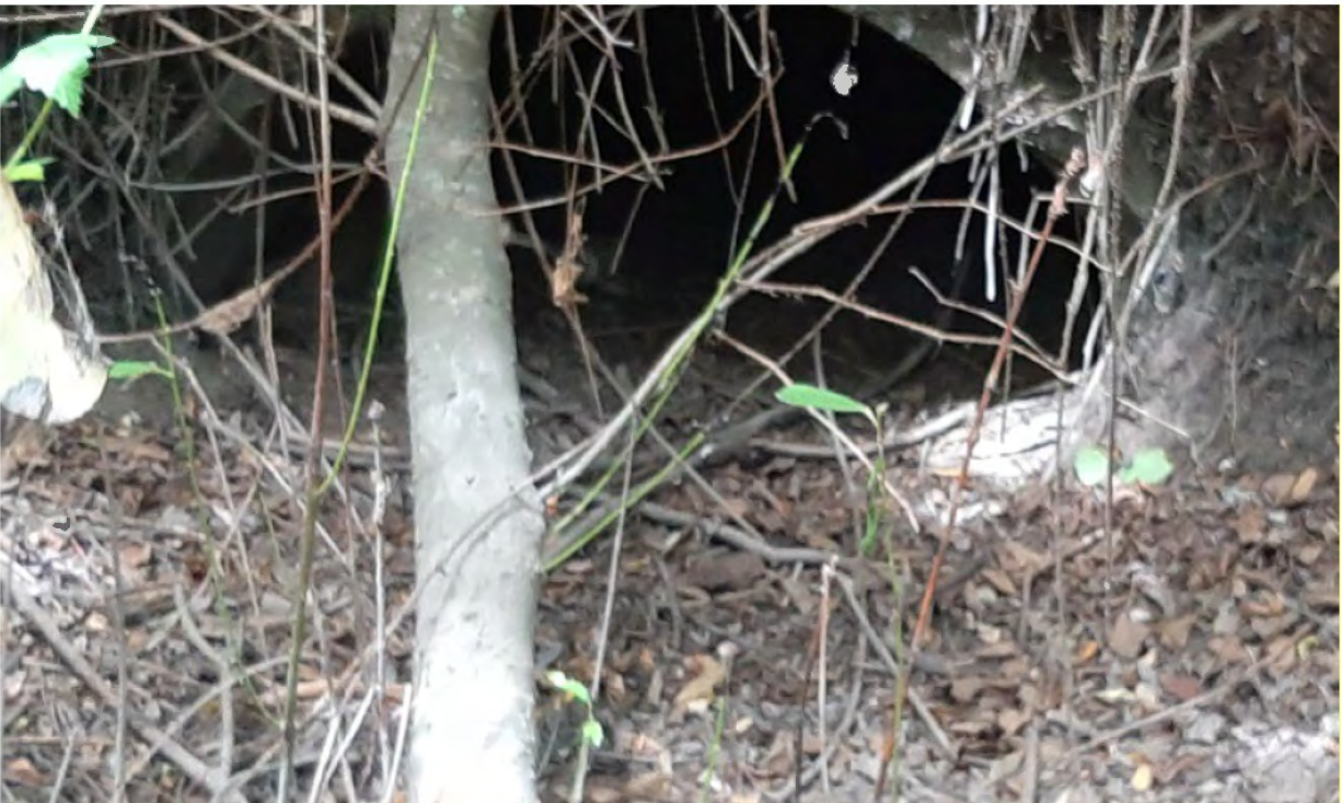
Photograph 20: Artificial aquatic feature- stormwater collection system near TP87. One of several stormwater culverts that drain into this feature. Photograph taken on June 29, 2022.
