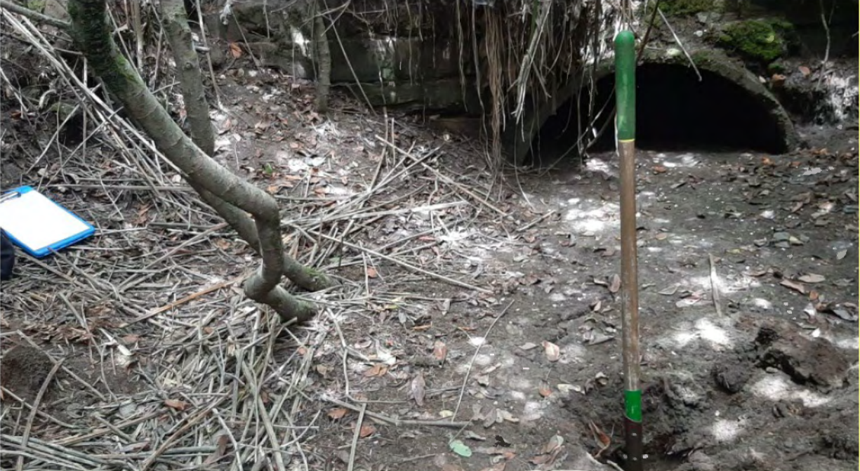
Photograph 19: Artificial aquatic feature- stormwater collection system at TP86. Culvert drains impervious surfaces formerly used for chip storage. Photograph taken on June 28, 2022.
