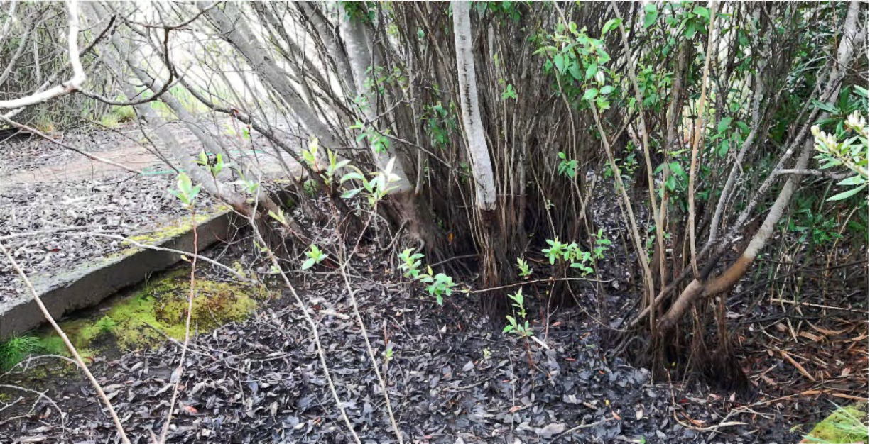
Photograph 16: Artificial aquatic feature at TP64 and TP65- an abandoned concrete vault and foundation that has developed into a three-parameter wetland.
