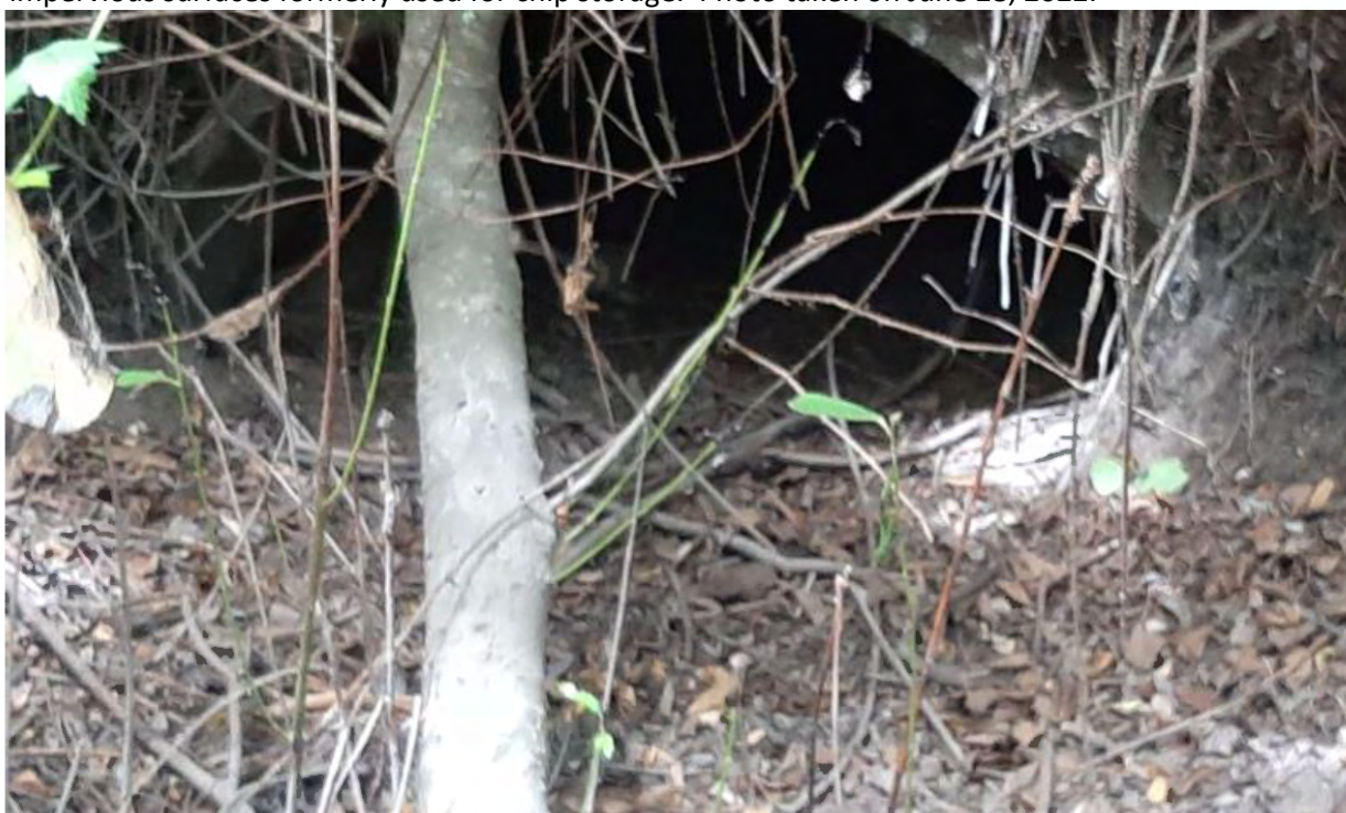
Photo 24: Potentially non-jurisdictional feature- stormwater collection system near TP87. One of several stormwater culverts that drain into this feature. Photo taken on June 29, 2022.
