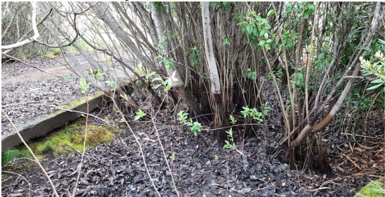
Photo 20: Potential non-jurisdictional feature at TP64 and TP65- an abandoned concrete vault and foundation that has developed into a three-parameter wetland.
