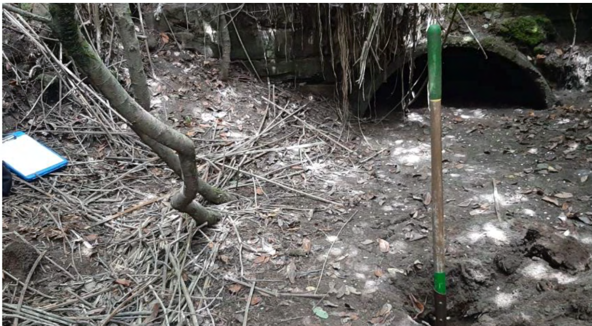
Photo 23: Potentially non-jurisdictional feature- stormwater collection system at TP86. Culvert drains impervious surfaces formerly used for chip storage. Photo taken on June 28, 2022.
