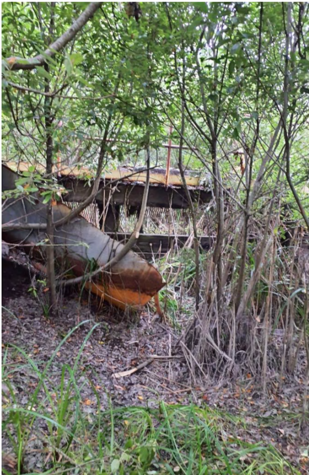
Photo 26: Potentially non-jurisdictional feature-stormwater collection system near TP88, near one of weirs before the entrance to Humboldt Bay. Photo taken on August 2, 2022.
