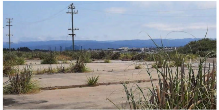
Photo 14: Concrete with some ruderal vegetation growing in cracks, typical within the southern portion of the study area, looking east. Photo taken July 29, 2022.
