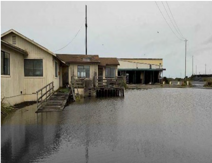
Photo 60: Abandoned buildings with standing rainwater on pavement. Photo taken April 13, 2022.
