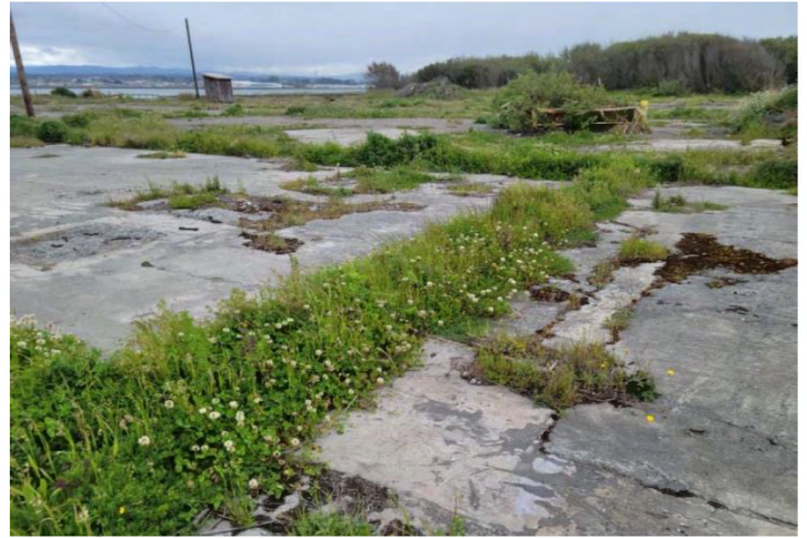
Photo 10: Concrete foundation with ruderal vegetation growing in cracks. Note ruderal vegetation over asphalt in background and coast willow/Sitka willow thicket beyond. Photo taken May 6, 2022.
