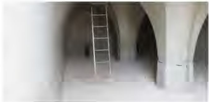
Interior of filter chamber
