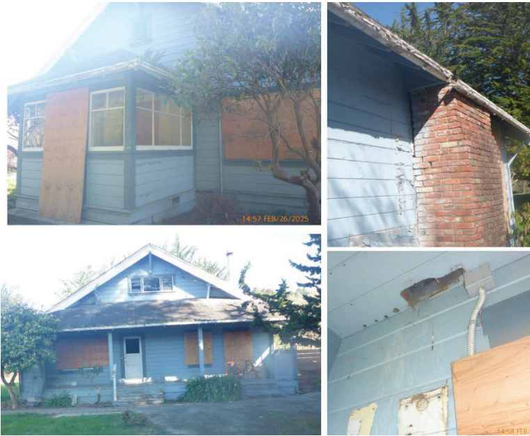
Figure D-8. Area 1 house view from the exterior with gap between the chimney and the house (top right) and access to the attic (bottom right).
