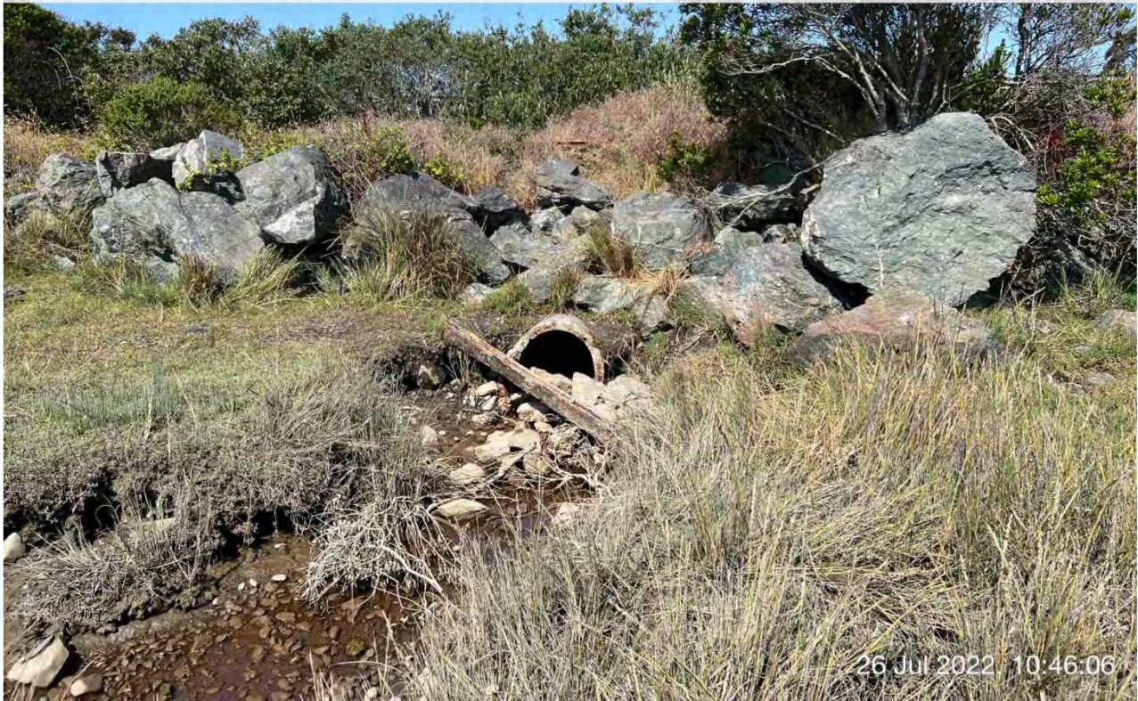
Photo D-5. View of a culvert on the shore of Humboldt Bay. No rare plants were observed at this location.
