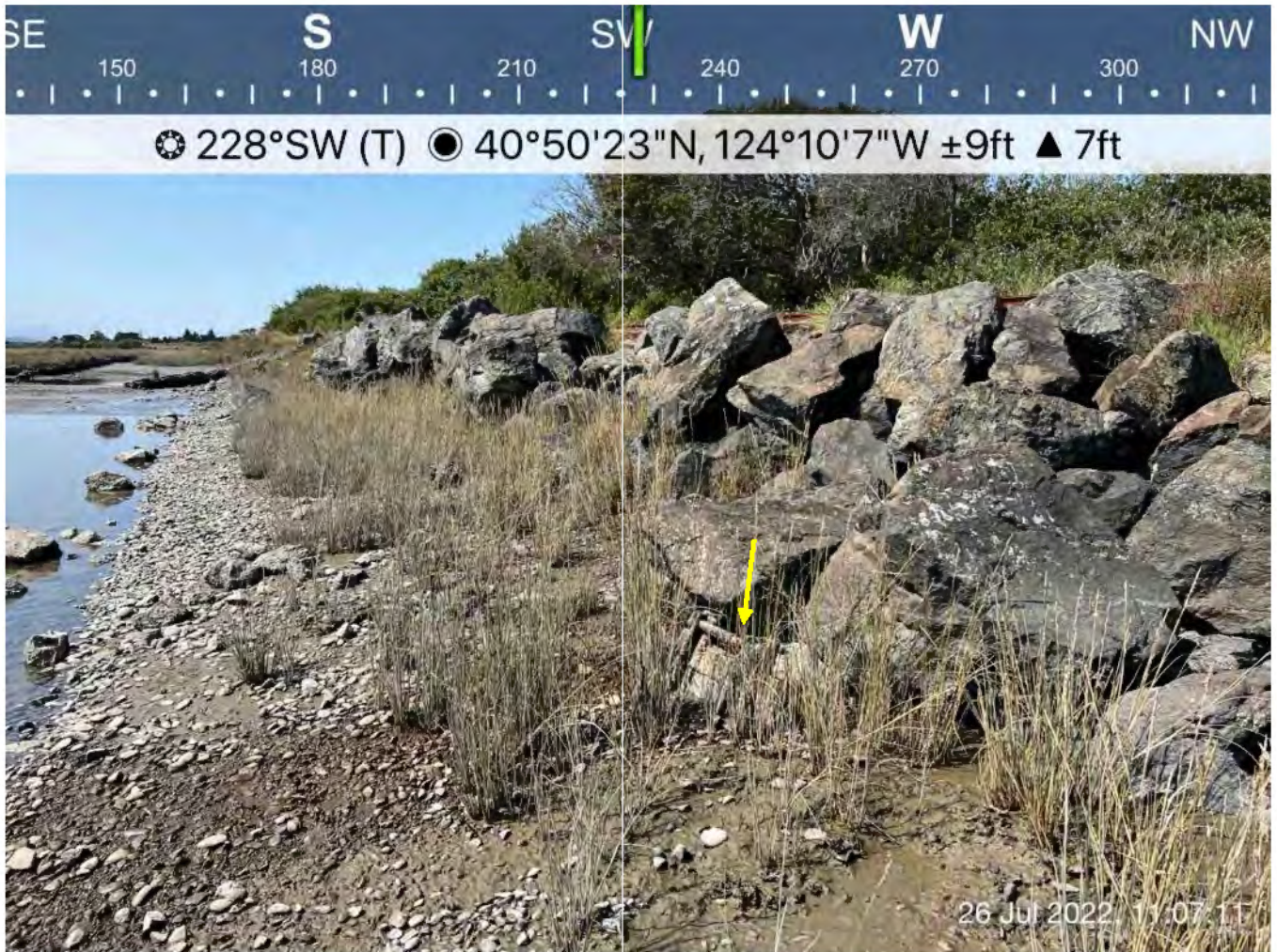
Photo 7. Southernmost culvert (below yellow arrow) on the shore of Humboldt Bay in estuarine marine wetland, July 26, 2022.
