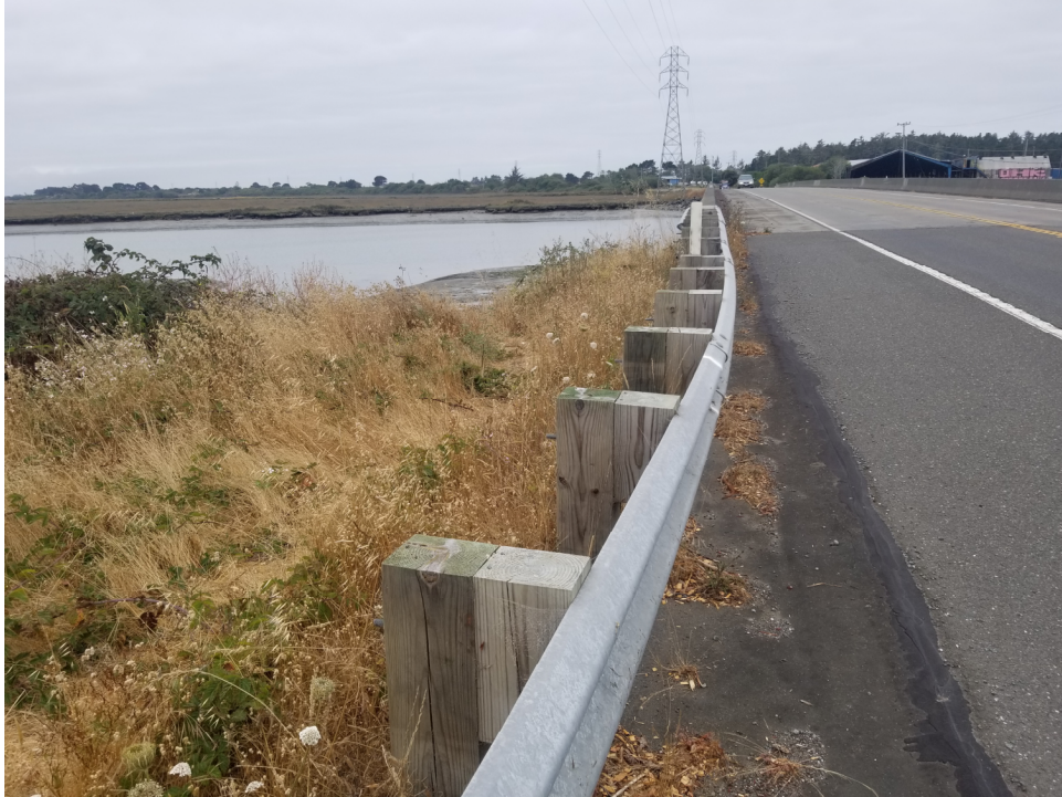
View of south Side of the Mad River Slough looking west towards the Sierra Pacific Saw Mill
