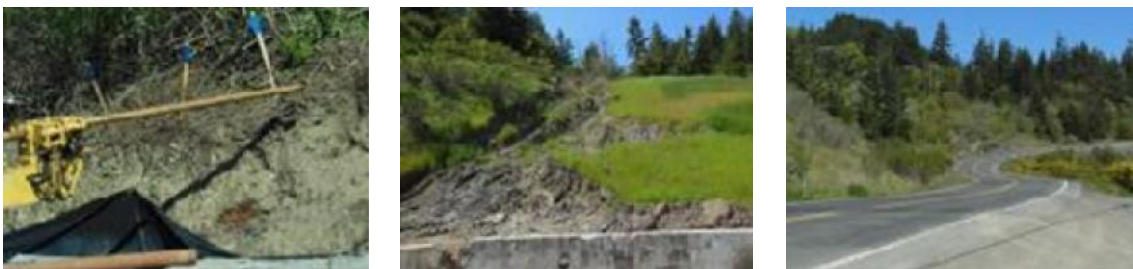
Figure 5 – Photos of Active Landslides Near Proposed Rail Routes
