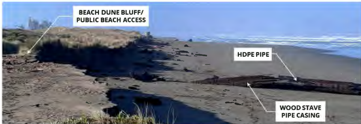
Photograph 3. Ocean outfall pipe daylighting onto beach. View looking south-southwest. Taken March 14, 2024, 9:20 AM. Approximate tide level -0.23 feet, NAVD88.
