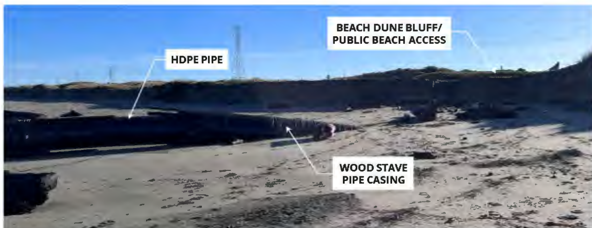
Photograph 2. Ocean outfall pipe daylighting onto beach. View looking northeast. Taken March 14, 2024 9:11 AM. Approximate tide level -0.15 feet, NAVD88.
