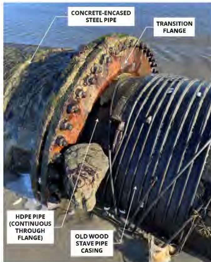
Photograph 5. Ocean outfall pipe transition flange closeup. View looking north-northwest. Taken March 14, 2024, 9:35 AM. Approximate tide level -0.25 feet, NAVD88.
