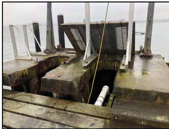
Image 5: Existing concrete sea-chest and screens at the Red Tank Dock. This sea chest will continue to be utilized; the screens will be replaced.
