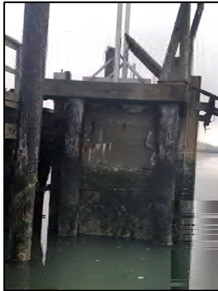
Image 6: Existing concrete sea-chest at the Red Tank Dock. This sea chest will continue to be utilized.
