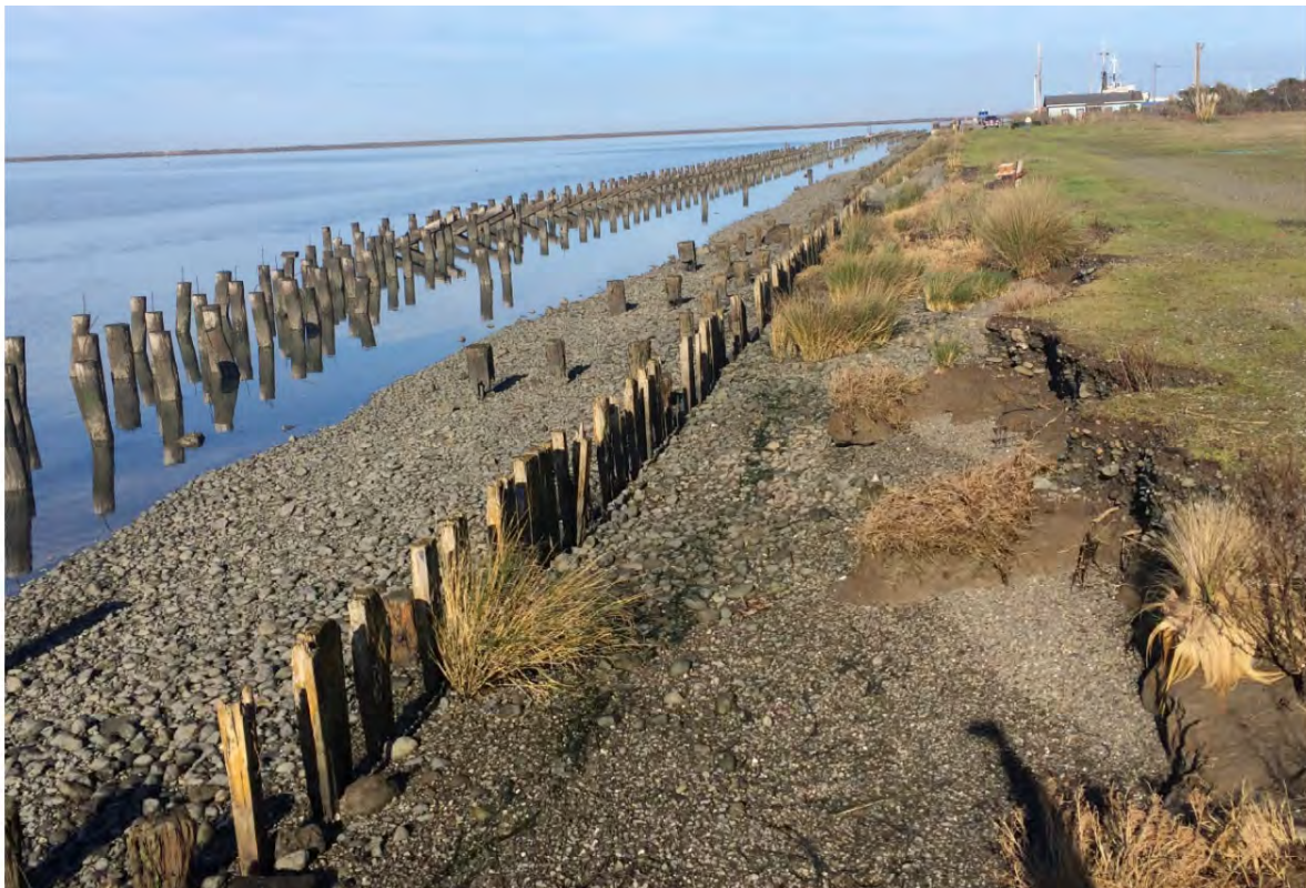
Figure 2. Photo of representative shoreline erosion at project site. Photo source: Stillwater Sciences, 2016
