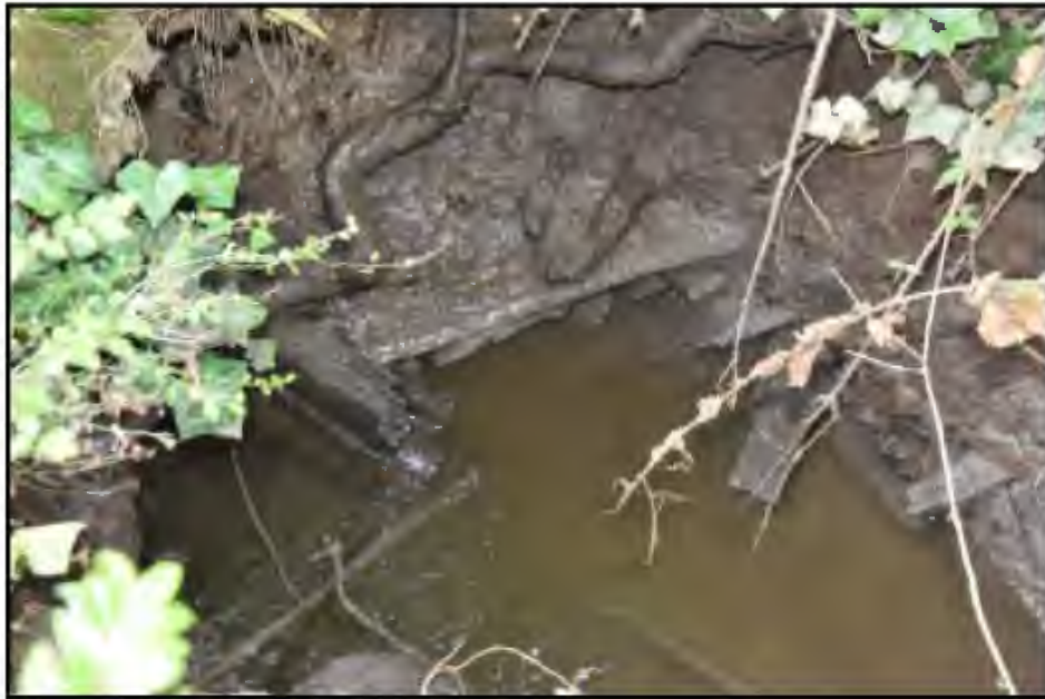
Figure 2.3-3. Redwood Timber Foundation Proposed for Removal
