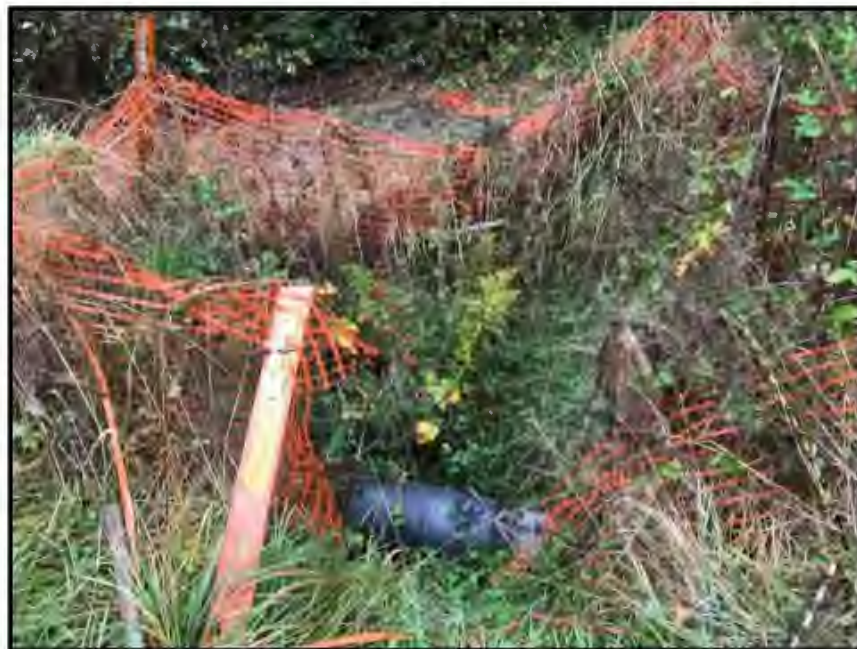
Figure 2.3-1. Sinkhole and Pipeline Exposure at RT-102 Project Site
