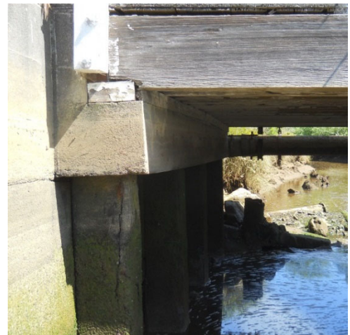
Figure 1: Vertical Cracking on Piles
