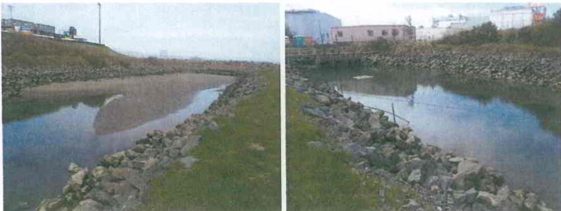
FIGURE 6 The Discharge Canal Looking toward the North End and Outfall Structure (left photo) and South View (right photo).
