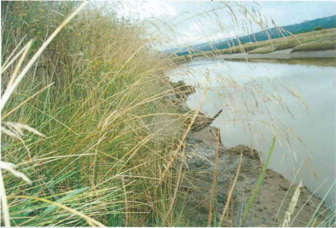
Eroding levee: looking down at levee face from the top of the levee
