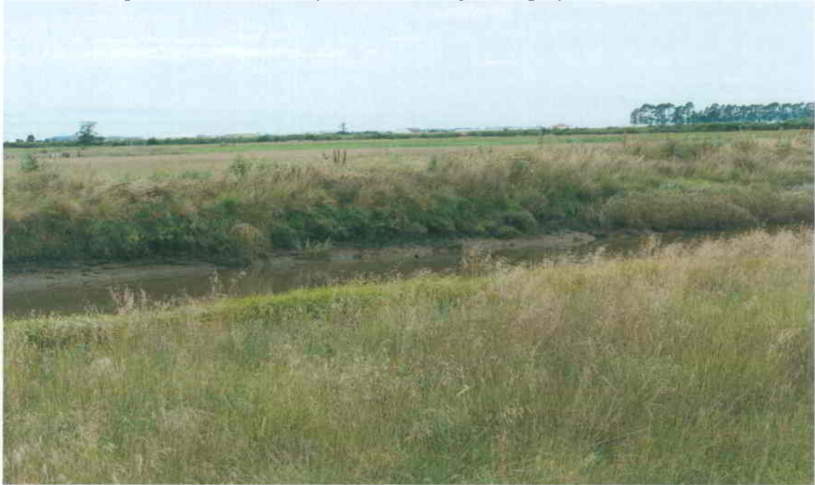
Downstream portion of the eroding Levee: looking at the project area from across the slough
